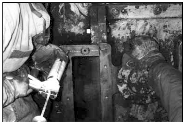
Loctite® 5900™ RTV Silicone Flange Sealant is applied as a final seal to the inspection cover of the paper machine gear section. All marked bolts are sealed and secured with Loctite® 243 Removable Threadlocker.
