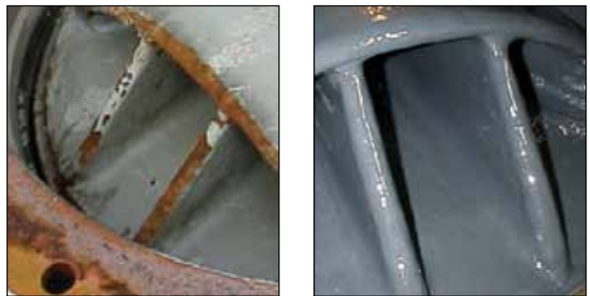
The corroded butterfly valve before and after repair
