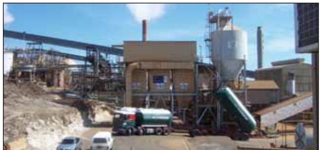
Bag house is subjected to extreme heat, moisture, and chemical attack
